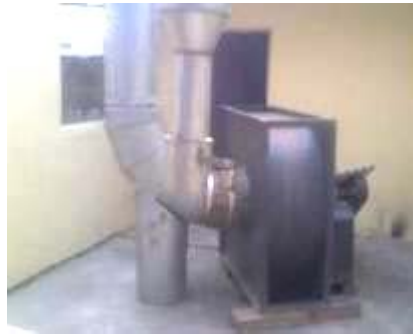
Discharge port and the main fan unit
